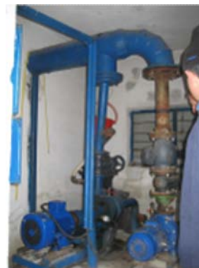
Noile pompe instalate
