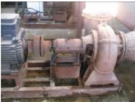
Pompe de spalare in contracurent
