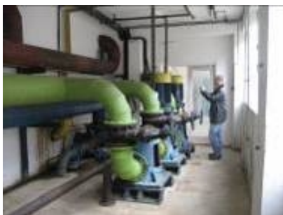
Pompe de spalare in contracurent
