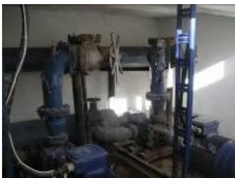
Noua pompa instalata a
