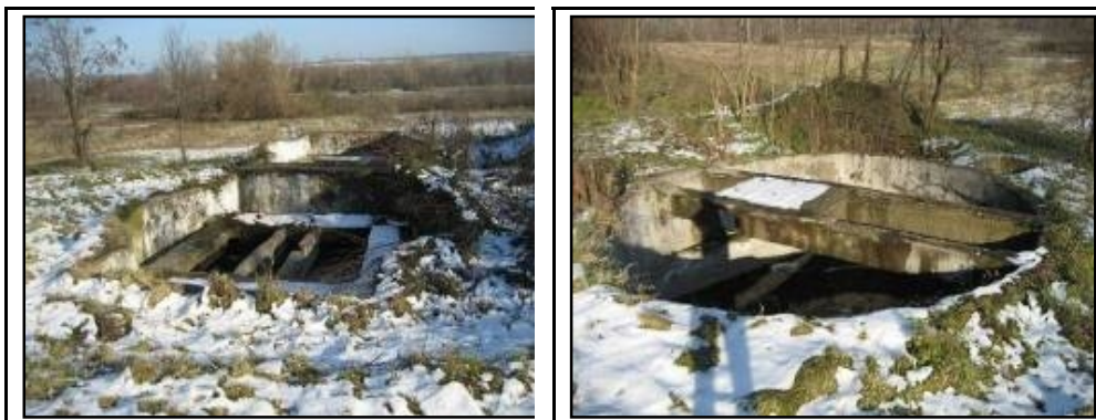
Figura2.10-55: Separator nisip defect Figura2.10-56: Rezervor de aerare defect
