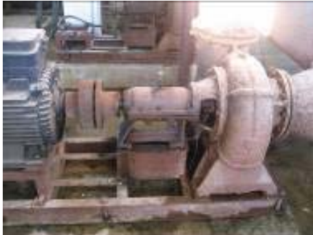
Pompe de spalare in contracurent
