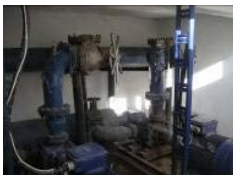
Noua pompa instalata a
