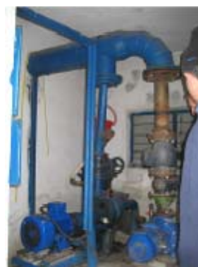
Noile pompe instalate
