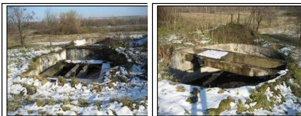
Figura 2.10-25: Separator nisip defect Figura 2.10-26: Rezervor de aerare defect
